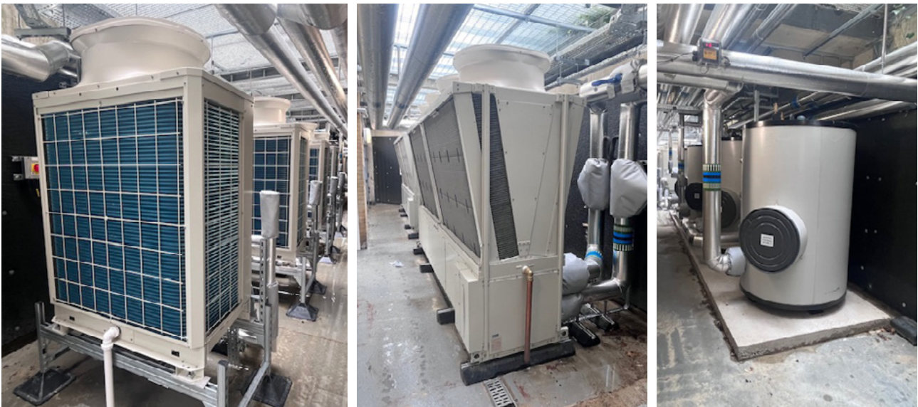
Saïd Business School project (images from left) air source heat pump providing hot water to the site, air source heat pumps providing heating, hot water tanks storing heated water from heat pumps (two tanks for hot water, two tanks for heating).
